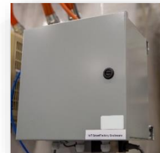
IIoT PLC Enclosure
