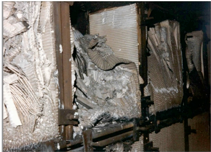
Figure 3. Water Damage to Filters Following a Fire
