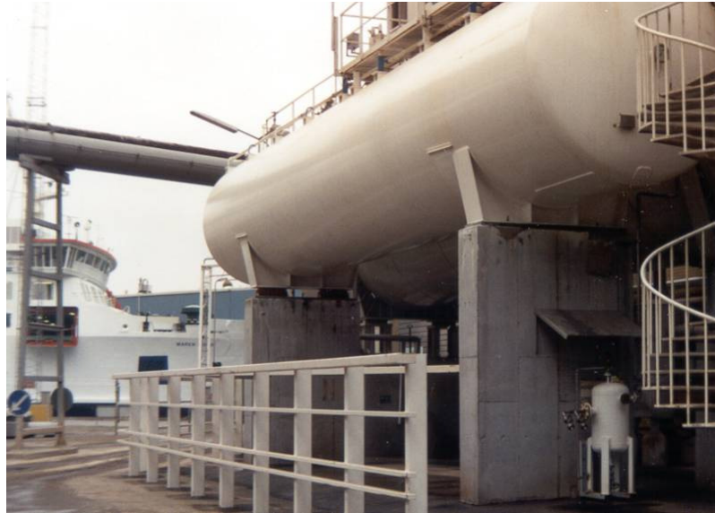
Figure 8.5 Highly protected ammonia storage vessel
