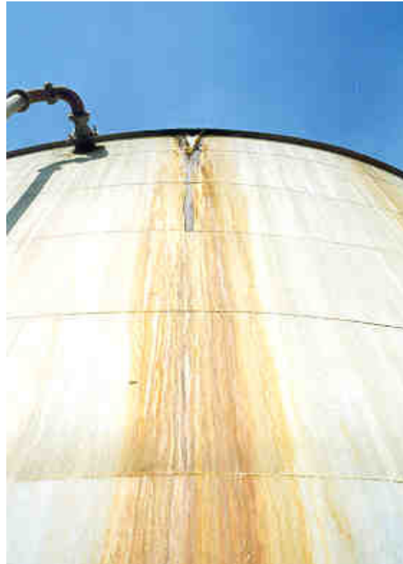
Figure 9.3 Leak from an acid tank due to corrosion at the acid, wall, air interface
