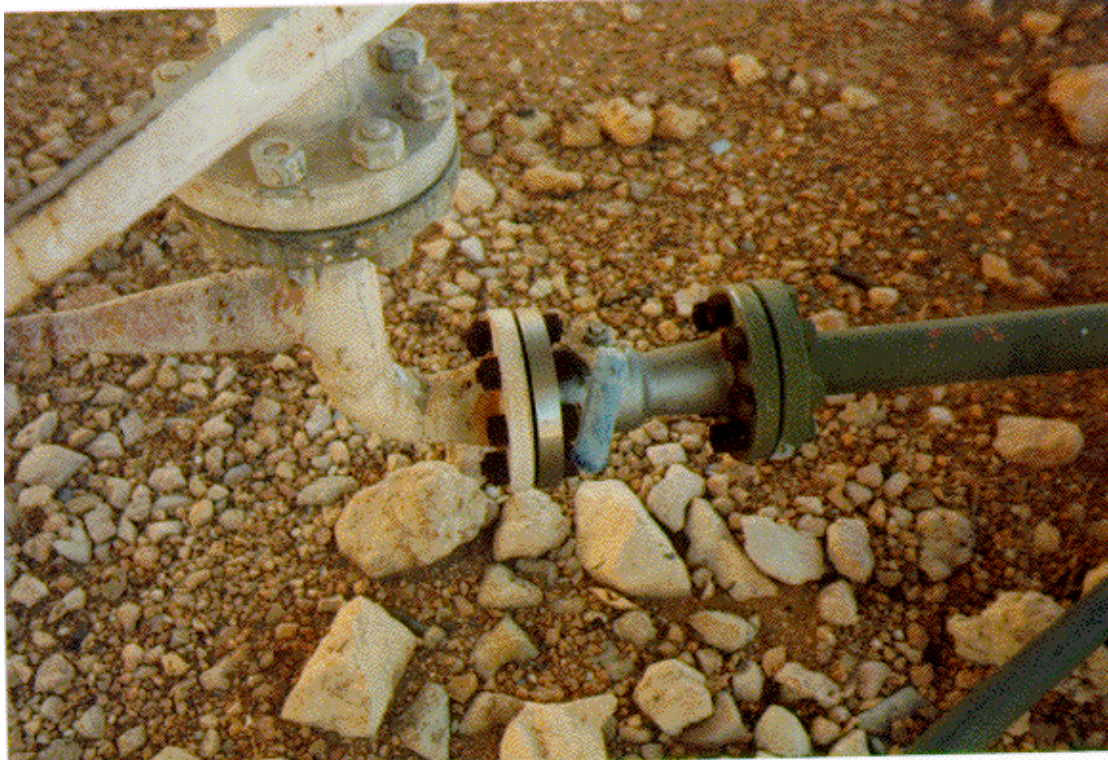
Figure 7.2. Galvanic corrosion on carbon steel bolts in a stainless spool piece
