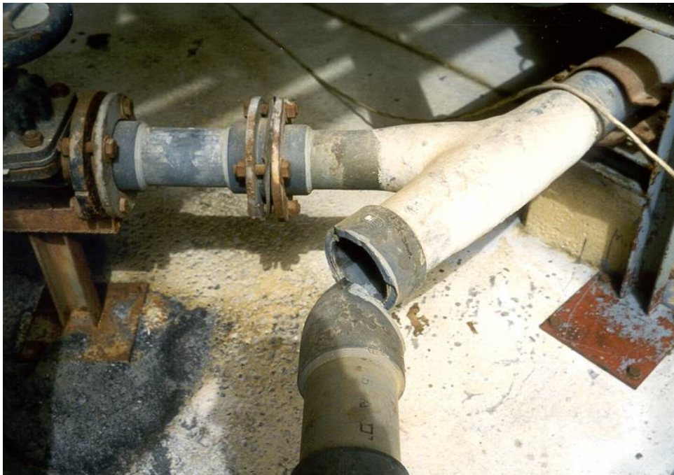
Figure 7.6. Pipe elbow broken by impact (PVC pipe)
