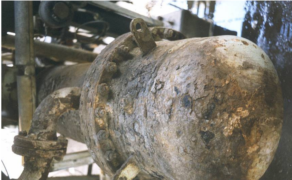
Figure 19.3 Heavy external corrosion on a heat exchanger due to the use of an external water drench to increase cooling capacity
