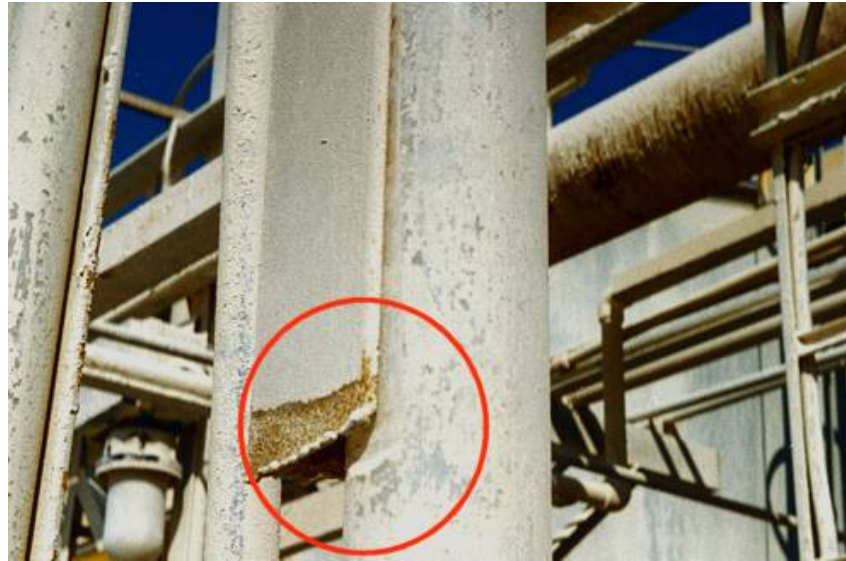
Fig. 7.4 High quality PVDF pipe damaged by fretting
