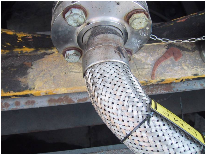
Figure 11.5 A poor use of a hose, with a very tight bend at the coupling
