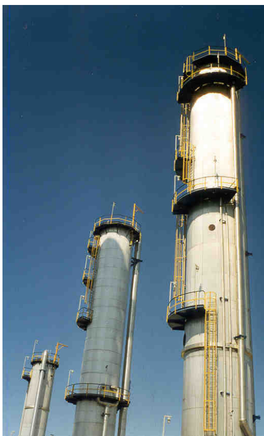
Figure 18.1 Distillation columns in a BTX plant
