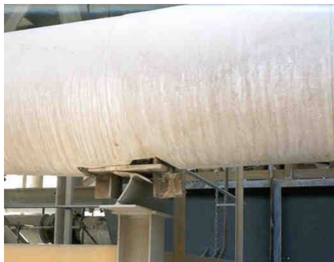
Figure 7.5 . Pipe support distortion arising from hammering during start-up
