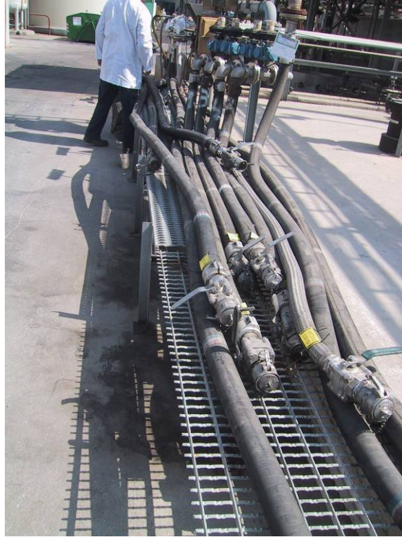
Figure 11.4 Properly stored hoses
