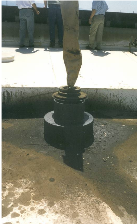
Figure 10.6 Splashing around a tank roof vent, due to filling with unstabilised crude.
