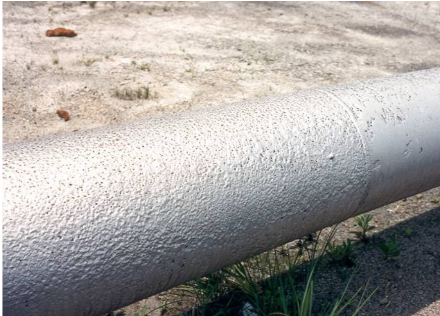
Figure 7.1. Pipe with very heavy pitting corrosion, after painting. Note that two adjacent pipe sections had very different susceptibility to pitting corrosion, possibly due to the corrosion occurring under different conditions in storage
