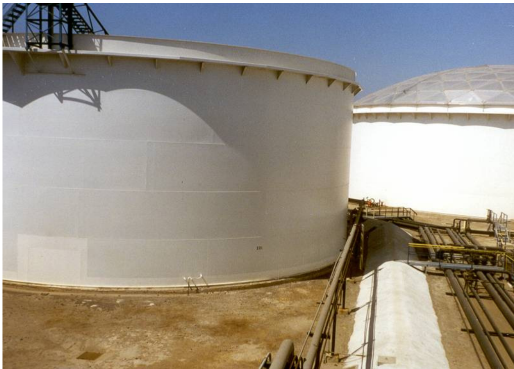
Figure 10.1.2 Floating roof tanks. The tank at the rear has a sheet plastic dome to reduce vapour loss.
