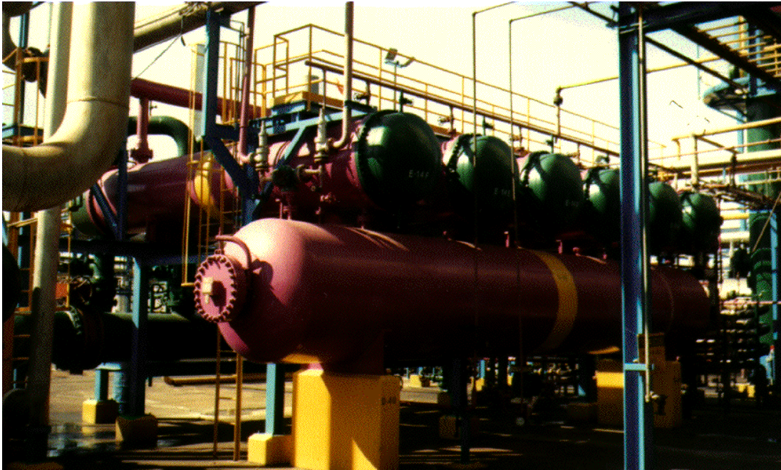
Figure 8.7 In process pressure vessels, ammonia plant
