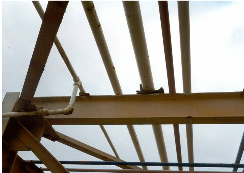
Figure 7. 8 Pipe supported on an old glove. Eventually the glove will rot away.
