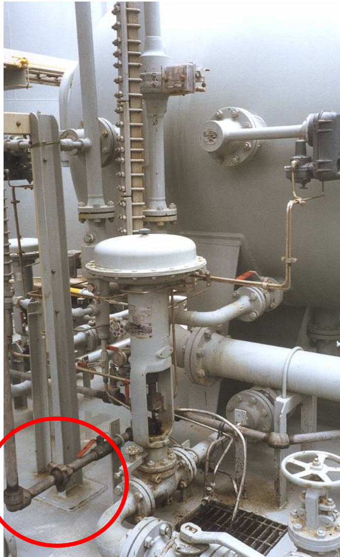
Figure 7.17 Small bore fittings alongside flanged connections
