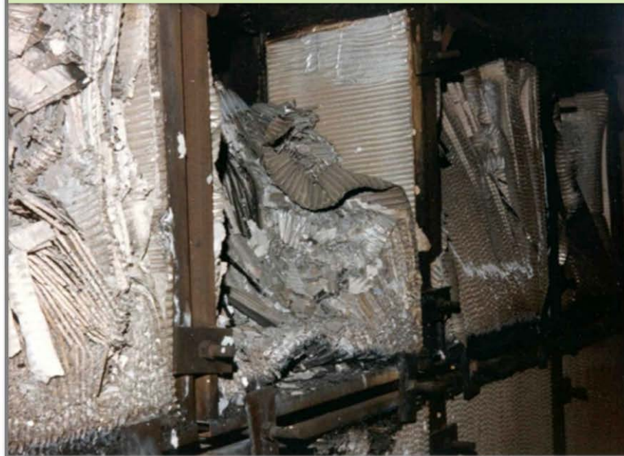
Water damage to filters following a fire
