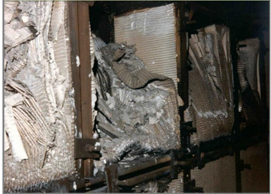
Water damage to filters following a fire
