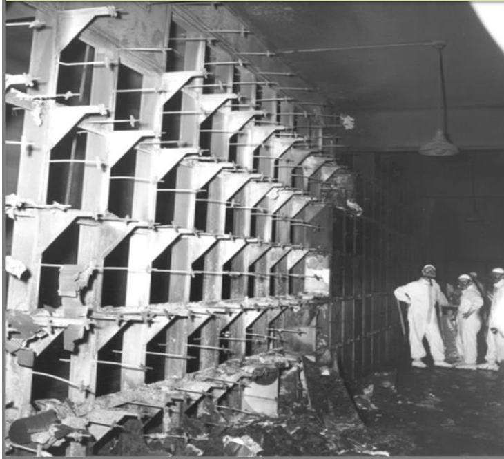
Destroyed filter bank after a fire
