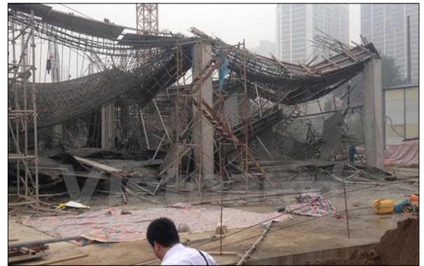
The scene of a scaffolding collapse at the construction site of Toyota Mo Lao Ltd in Hanoi killed three people and injured three others. – VNA/VNS Photo
