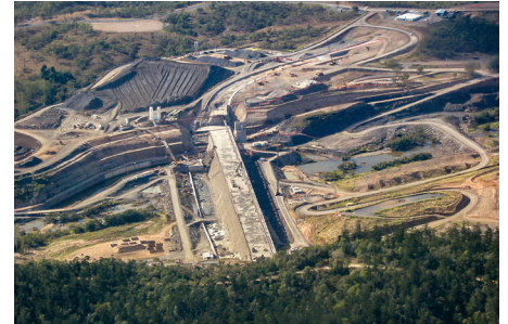
Paradise Dam was only built 19 years ago, yet it was supposed to stand for a century. Image courtesy of Rod Savidge.
