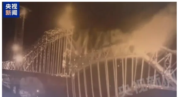
A screengrab from video published on Aug. 22, 2025 by Chinese state television shows a portion of the under-construction Jianzha Yellow River Bridge, a key project of the Sichuan-Qinghai Railway in Jianzha County, Qinghai Province, China, collapsing. The incident killed at least 12 people, according to China's state-run media.
