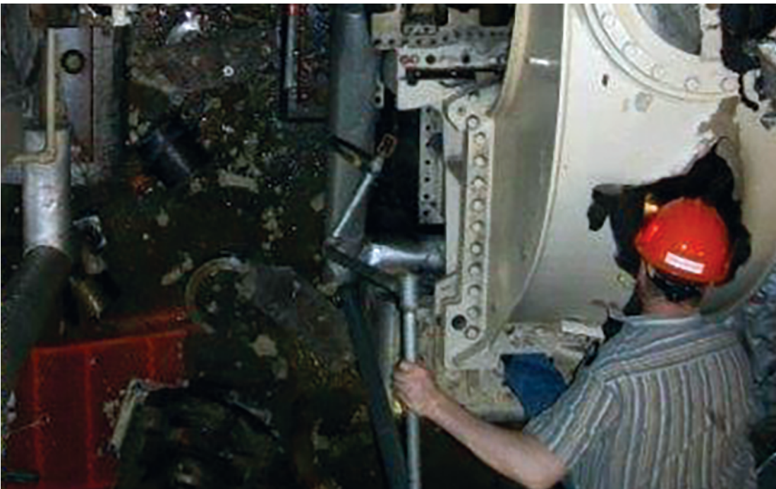
Figure 2. Wreckage on the exhaust hood and low-pressure end bearing
