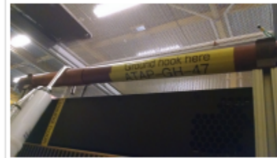
Figure 22b. Example of showing each ground stick placement instructions and photo into the equipment specific LOTO procedure to reduce human error.
