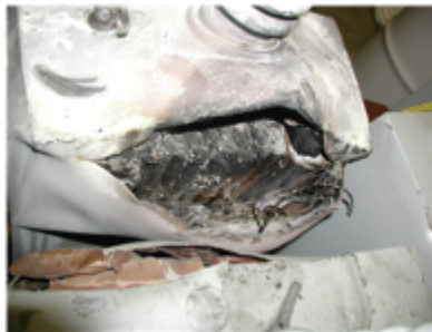
Figure 8. A failed capacitor.
