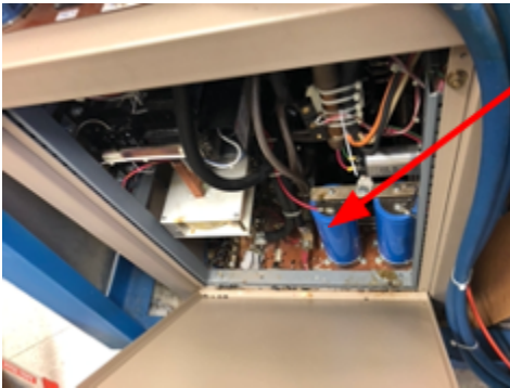
Figure 4. Two capacitors embedded in a system.
