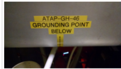
Figure 22a. Example of having steps with photos on the equipment specific LOTO procedure including instructions and displaying Ground Stick equipment ID.
