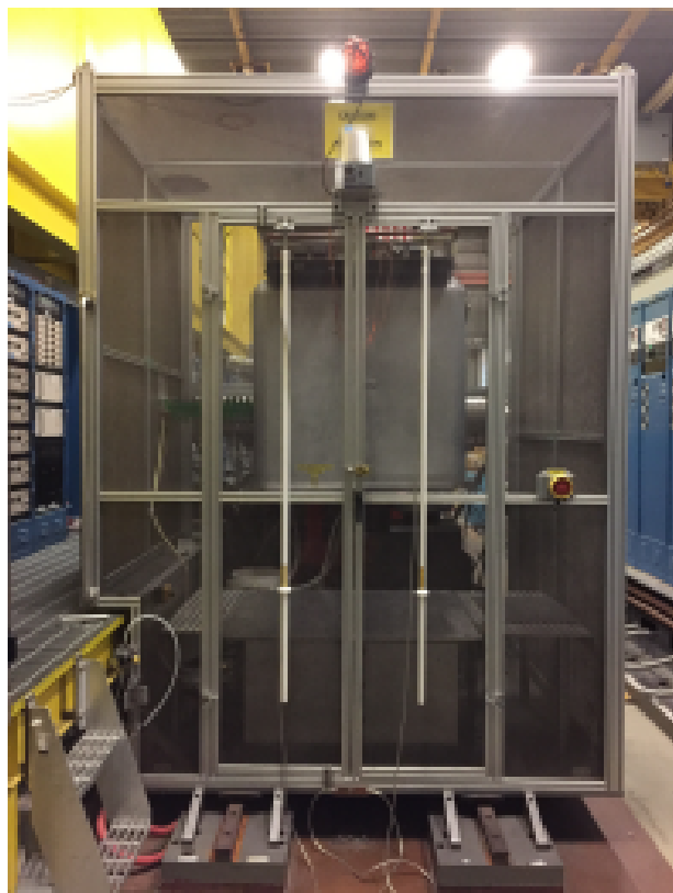
Figure 18. Photograph depicting the HV enclosure (cage) with custom grounding devices. HV dome can be seen through the front of the interlocked cage doors.
