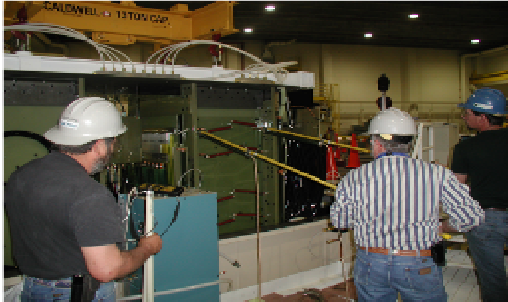
Figure 7. Example attaching a drain wire. Two workers on the right are holding soft shorting/ground sticks across a 1 MJ bank, while the worker on the left approaches with a drain wire.
