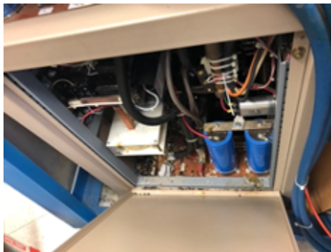
Figure 12. Two capacitors embedded in a system.
