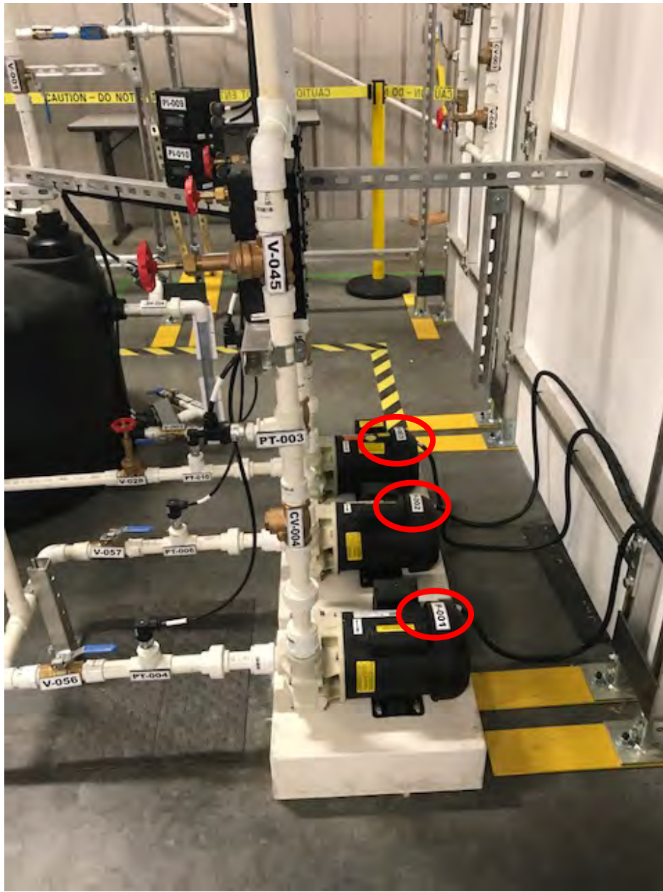
Example of side-by-side look-alike equipment with permanent equipment ID labels
