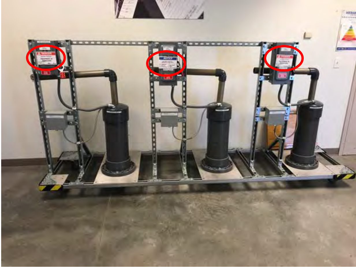
Example of side-by-side look-alike equipment indicating which ones are de-energized and under LOTO and which ones are energized
