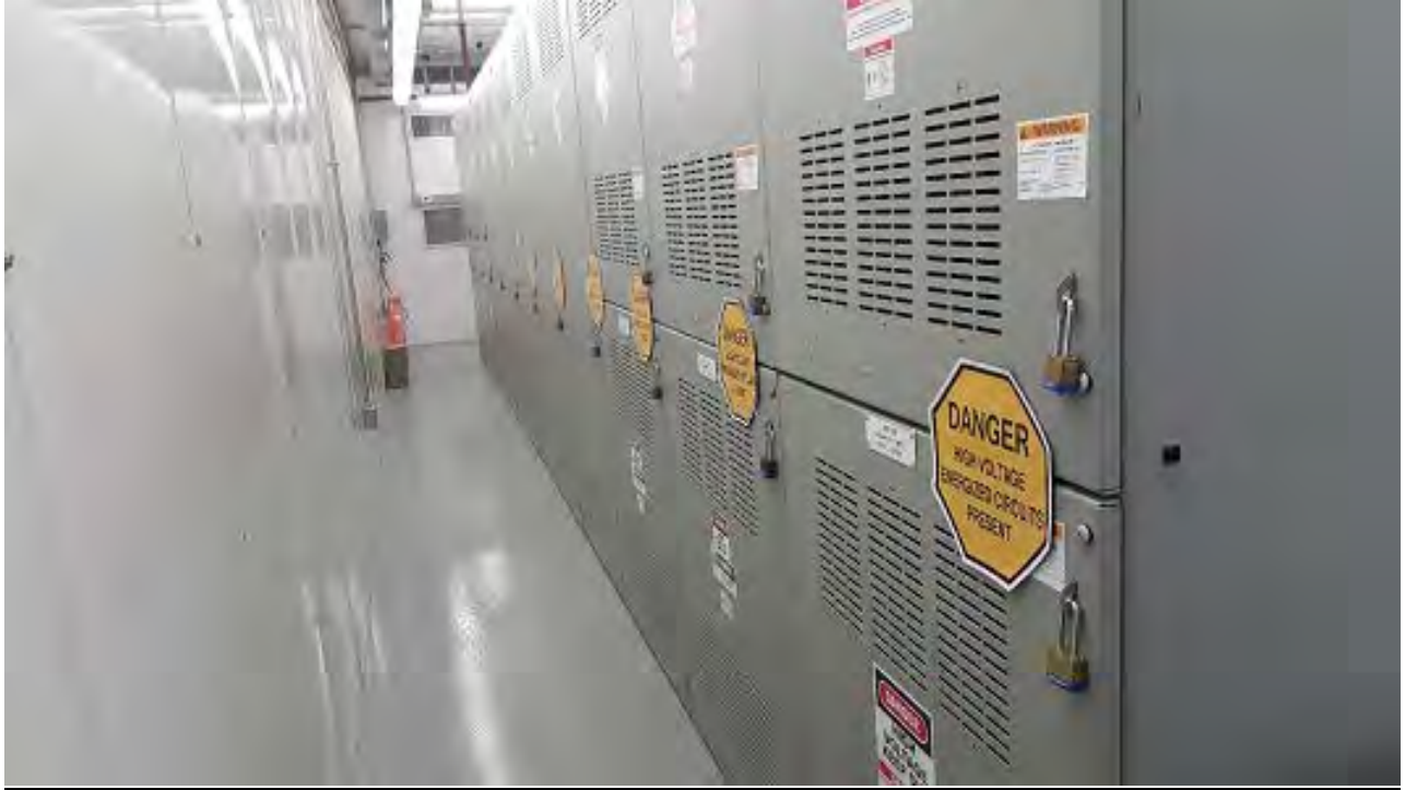
Example of installed magnetic signs sized appropriately for the equipment
