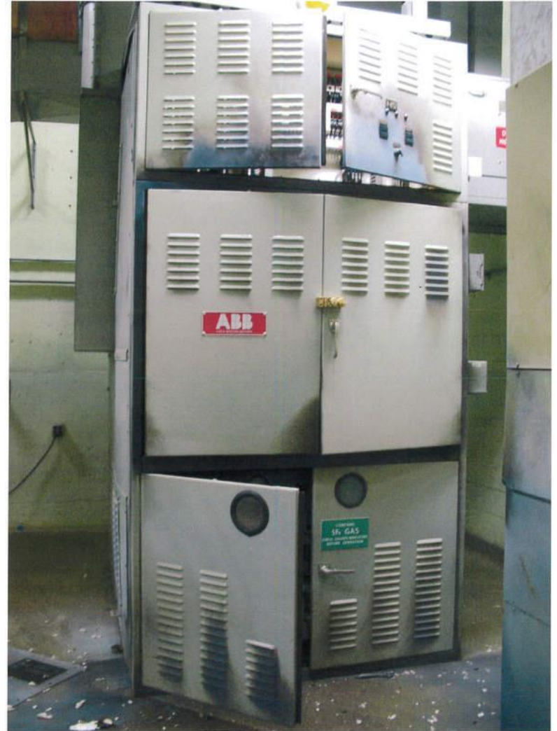
Generator Circuit Breaker
