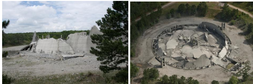
Cooling Tower (after)
