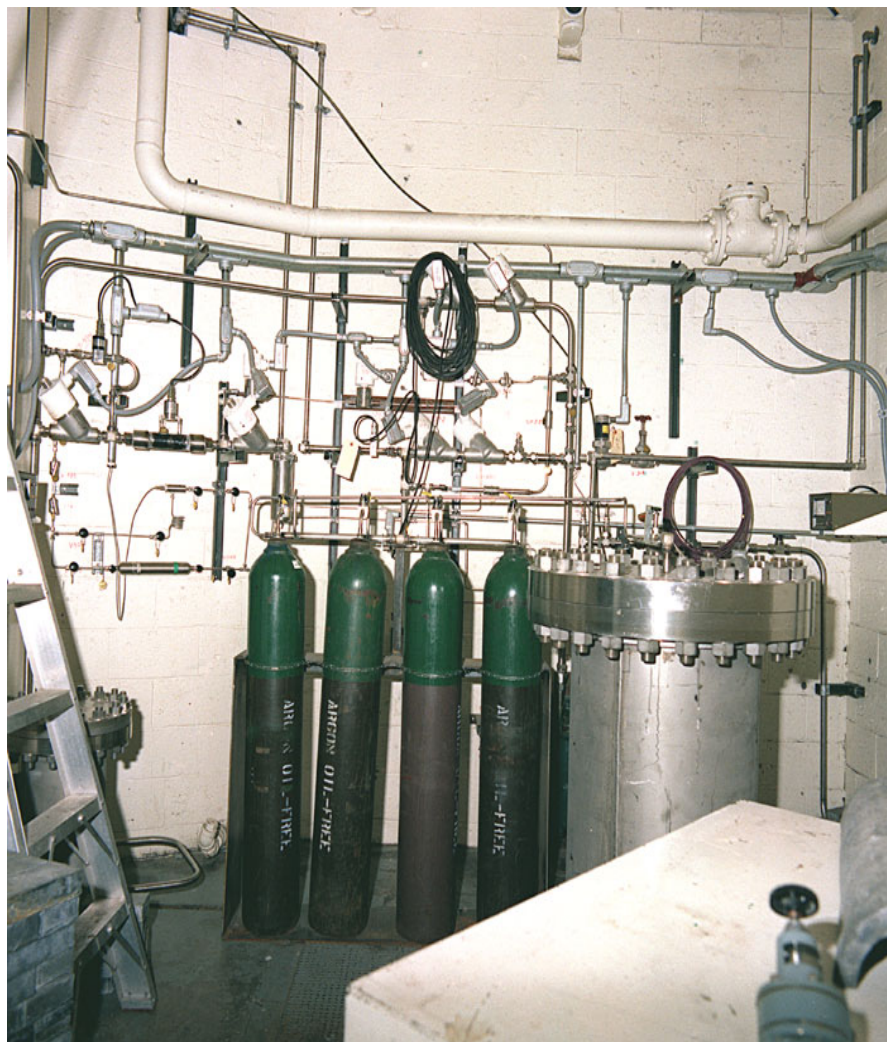
Figure 15. Annular gas system cubicle contents.
