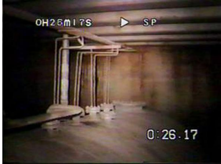
Figure 4. Top of Underground Waste Tank (from ERG 2006a)
