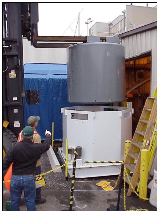
Figure 5. Typical Waste Package Suspended Over Shield (West Valley Demonstration Project Photo)
